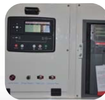
Control Panel & MCB
